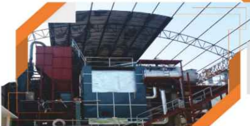
SHRI DAKSHINA MURTHY AGRO INDUSTRIES PVT. LTD., CHILAKAMARRI (TELANGANA) 10TPH, 17.54KG/CM 2
